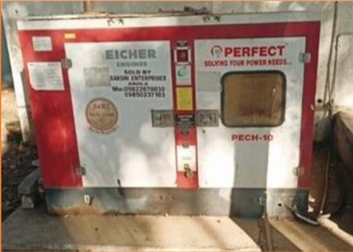
Power Backup Facility (Generator)
