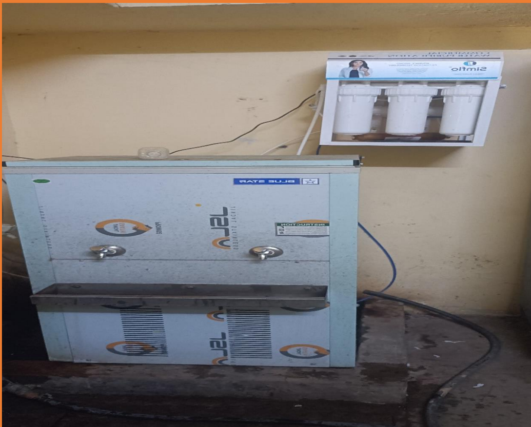
Water Cooler 3 (For Staff)
